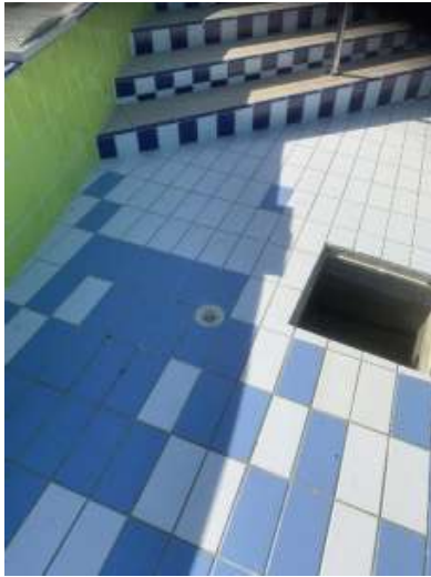
FLOOR RETURN THAT IS NOT CONNECTED
