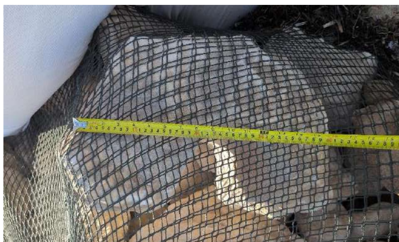
Figure 7. Oversized rock in existing bags.
