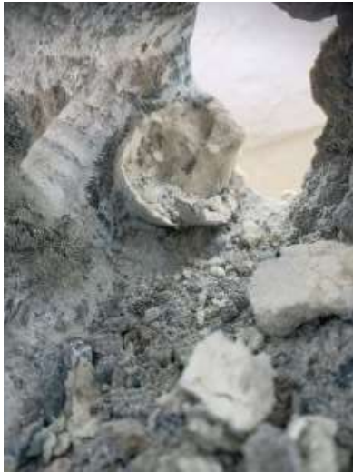
Showing one of the pipes that was not even capped off. And very little concrete cover into the gutters
