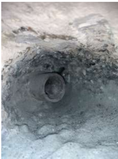
Pipe work that has been exposed in the steps
