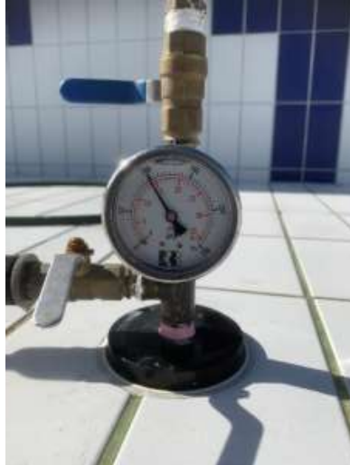
END OF TEST 25MT
