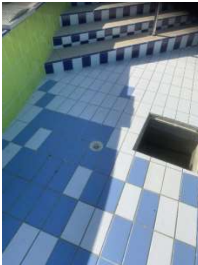
FLOOR RETURN THAT IS NOT CONNECTED
