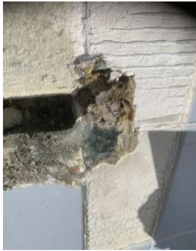
Showing bluey/black colour to concrete due to the pipes in the wall.
