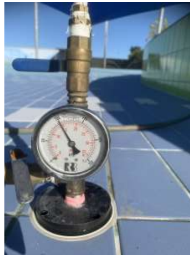
START OF TEST TO FLOOR RETURN THAT NOT CONNECTEED
